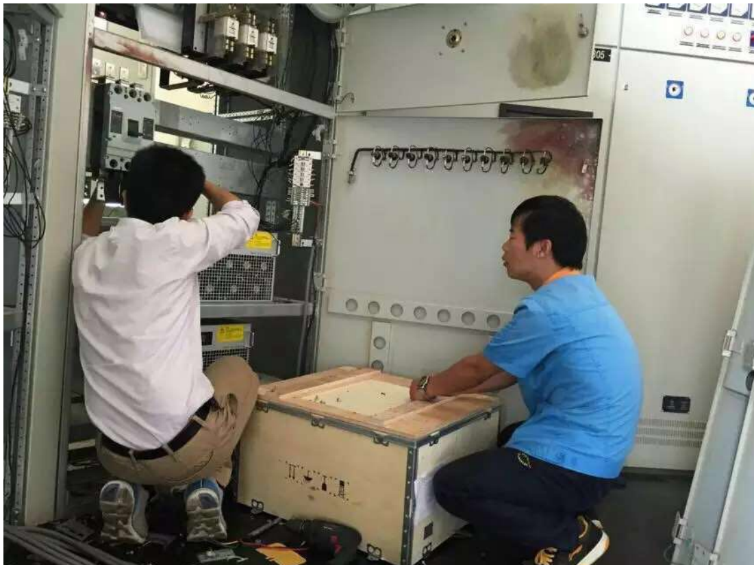
Figure 1(Cap bank explosion)
