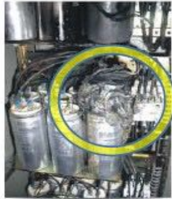
Capbank Overheat Fire risk
