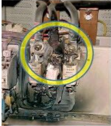
Busbar Joint Fire risk
