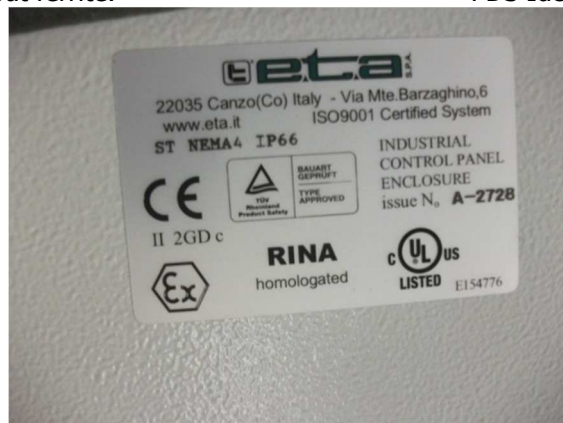
Enclosure identifier label.
